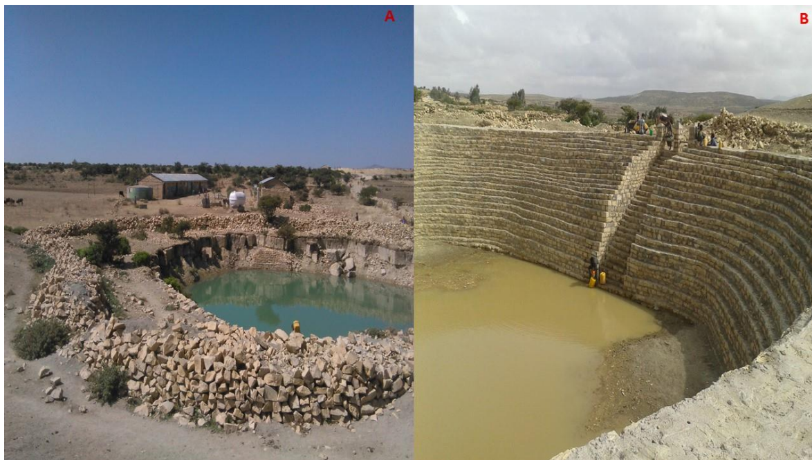
Figure 4. A hand-dug well close to a primary school in Tsuwanet with walls that easily collapse and also visible is a rainwater tank and a white storage tank close to the school building (Figure 4a). With financial support from World Vision International, a stone wall was constructed in May 2017 to protect walls from collapsing and also from livestock (Figure 4b).
